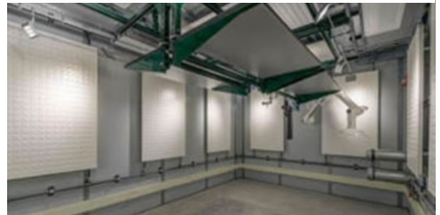
An ultra-low vibration chamber at ULVL with mass foundation, and RF shielding for the installation of a low vibration table.
