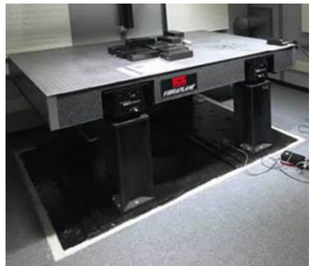
Customized Minus K Technology Negative-Stiffness vibration isolation table installed in the Ultra-Low Vibration Lab.
